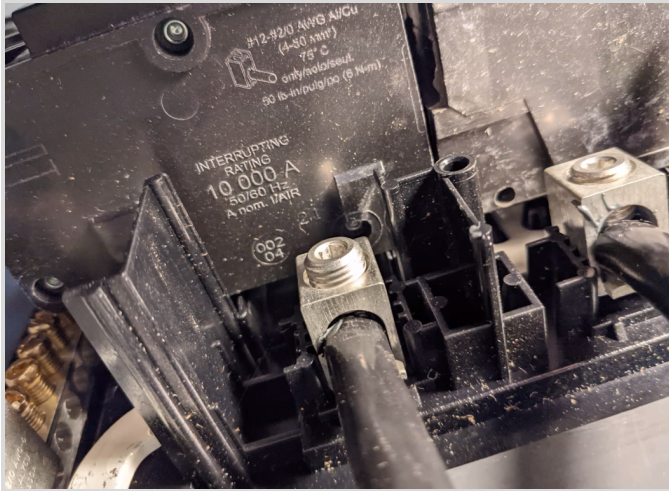
Connections on Curt's panel
