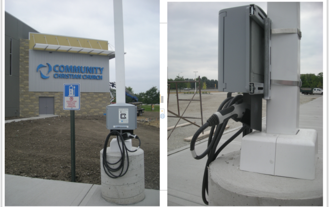
We have only had that one latch issue on the Clipper Creek since it was installed in 2014
