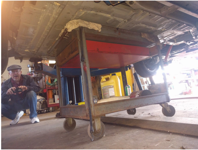
Bruce looks on as Bob's sturdy work cart holds the almost 800 pound battery pack. A series of bolts and ground-straps held the battery pack mechanically in place.
